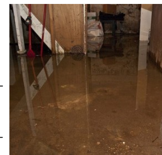
Picture of a flooded basement
